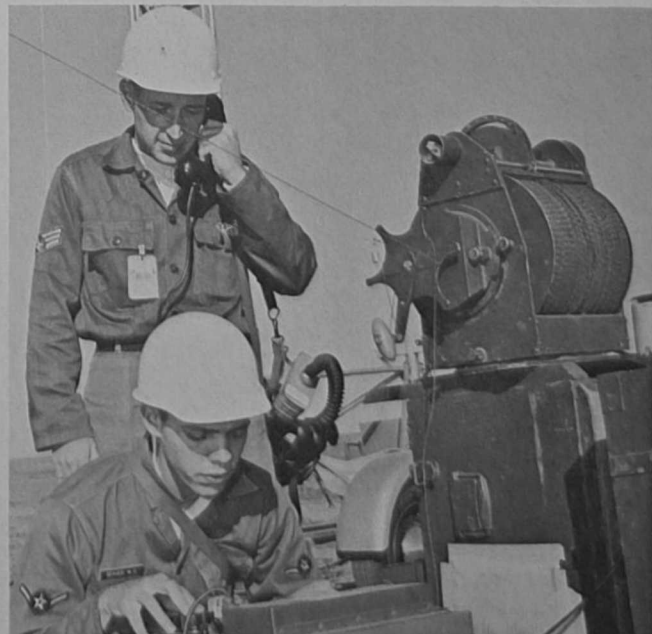
READINGS of atmospheric stability during installation and checkout of a Titan II missile site are taken by A3c Michael C. Seaver (foreground) and A1c Milton C. Scott, both of 6th Weather squadron (Mobile) on TDY at McConnell AFB, Kansas.
