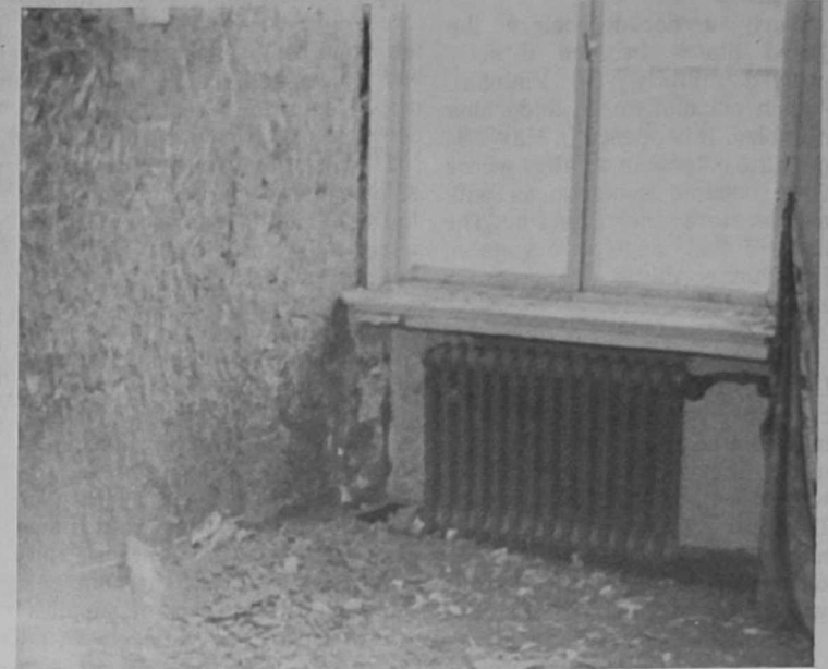
RUBBLE and filth was what the men found when they began construction of . . . . .
