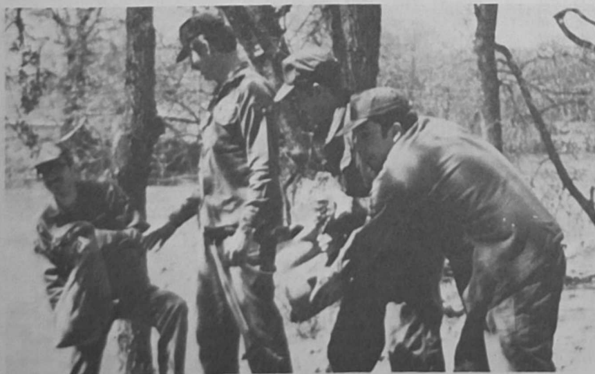
EVEN WITH no rain at the moment, Minot, ND's Souris River keeps rising—and the town is in danger. To fight the onslaught of water known to be coming, men of Detachment 21, 9th Weather Squadron, Minot AFB, help build then reinforce dikes to hold back the deluge. Left to right are A1Cs Todd R. Keupp, John Pennington, Brian W. Tenney and Lincoln A. Thorner. (U.S. Air Force photo)
