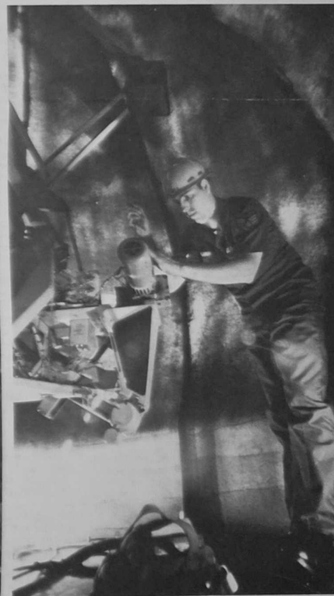
THE EERIE appearance of the FPS-77 weather radar radome takes on a television space program appearance. SSgt. Dave Graef adjusts the unit's antenna elevation drive system.
