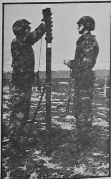
SSgt. K.G. Smith and Amn. Michael Pickerign secure the base of the GOLDWING antenna system during a training drill at Butts Army Air Field, Fort Carson.
