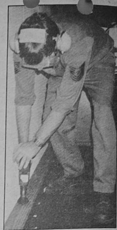
Pounding nails for Sharp Eagle the easy way, MSgt. Todd McIntosh fires a Ramset to set a wall support base. Working with self-help labor, det. members built a new area for weather data controllers and saved the Government nearly $20,000 by doing the work themselves. (U.S. Air Force photo)
